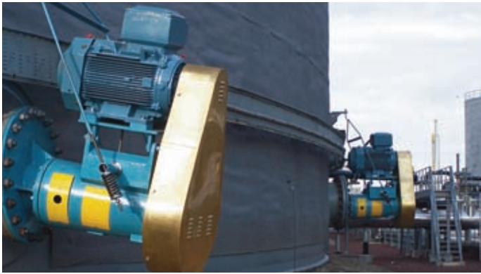
Fixed angle belt drive mixers including upward pointing unit on fuel oil blending in the Netherlands
