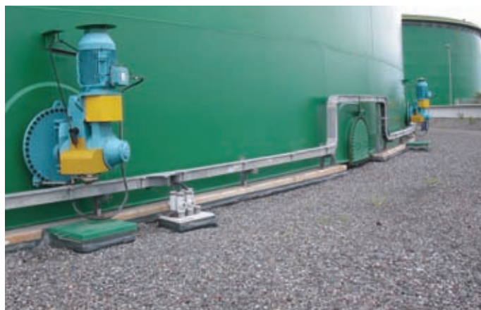
Gear drive swivel angle mixers on crude oil tanks in Ecuador
